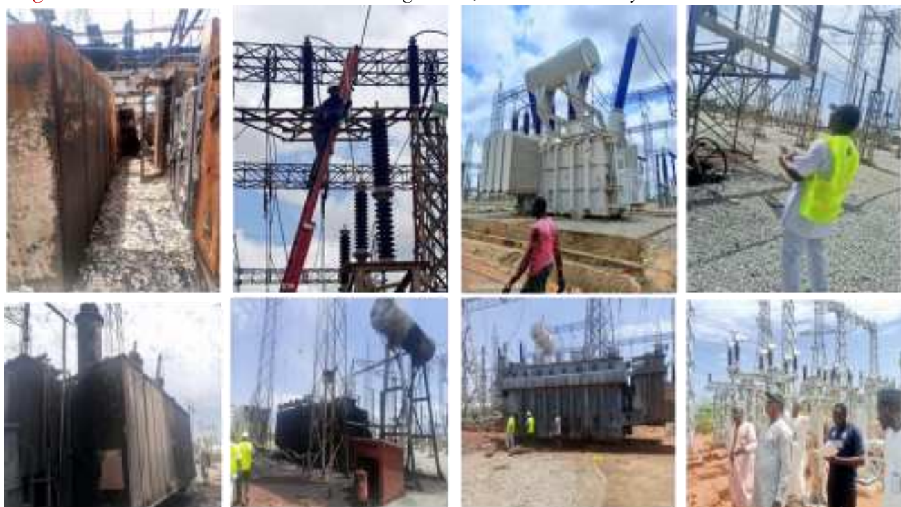
Figure 29: Investigation of Electrical fire at Transmission Sub-station Birni Kebbi, Kebbi State by NEMSA Technical team by the GM, Technical Inspectorate Services Department
