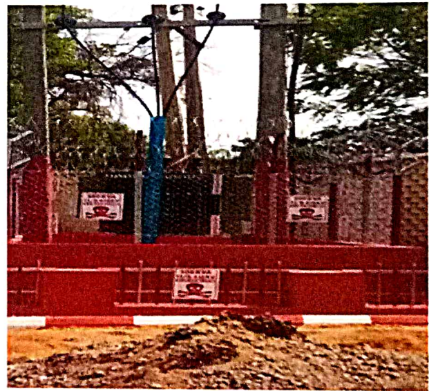
A well designed and constructed substation in GRA, Sokoto.
