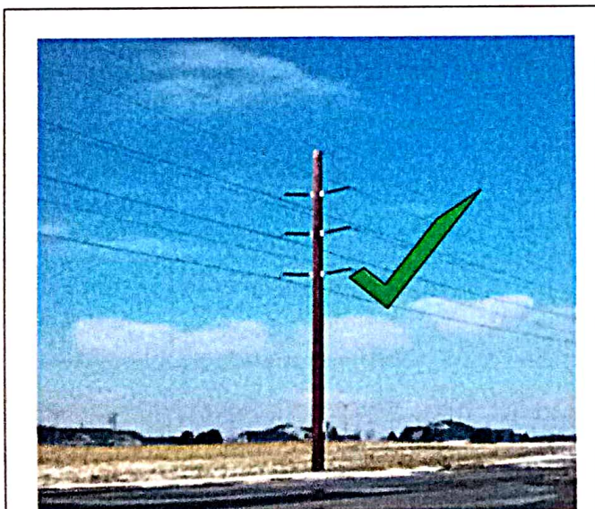
Good brackets that support proper spacing (separation) of circuits because the poles were specifically muddle for this type of construction.
