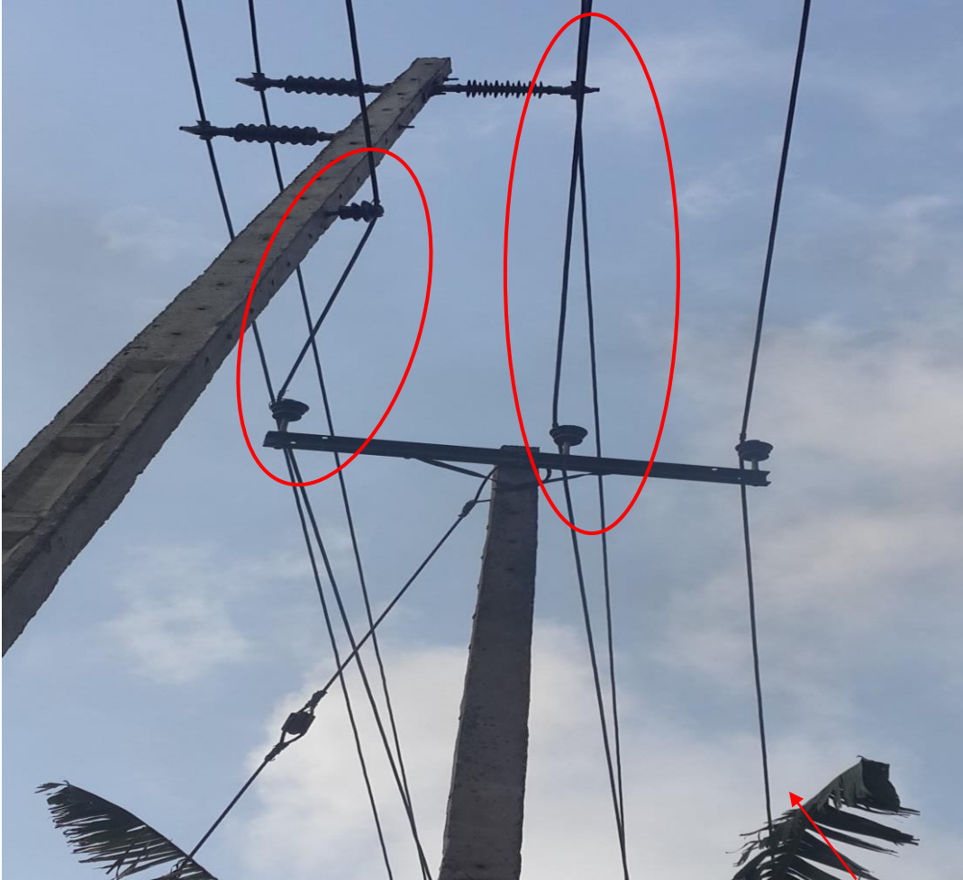
Unsafe construction with different lines on same pole, and different line construction types [Odogunyan, Ikeja Electric]
