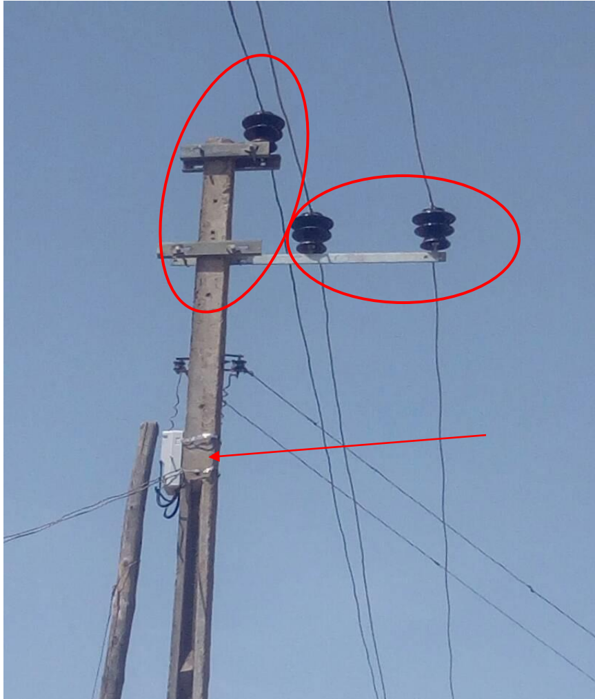
Unsafe construction with inadequate clearances and poor stability. [Jos Disco]
