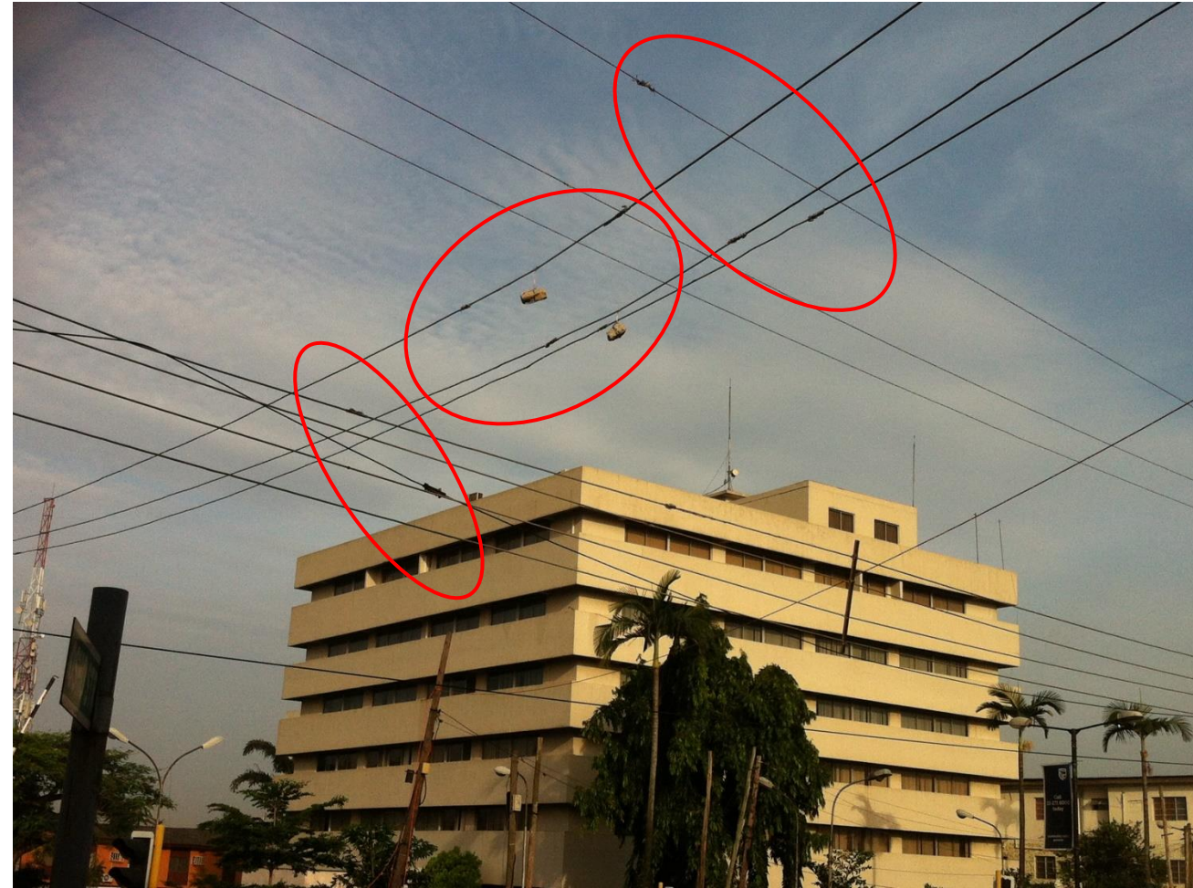
Pieces of concrete used to support conductors and multiple joints on HT lines at Opebi Road by Osho Street (Link Rd) Junction, Ikeja. [Ikeja Electric]
